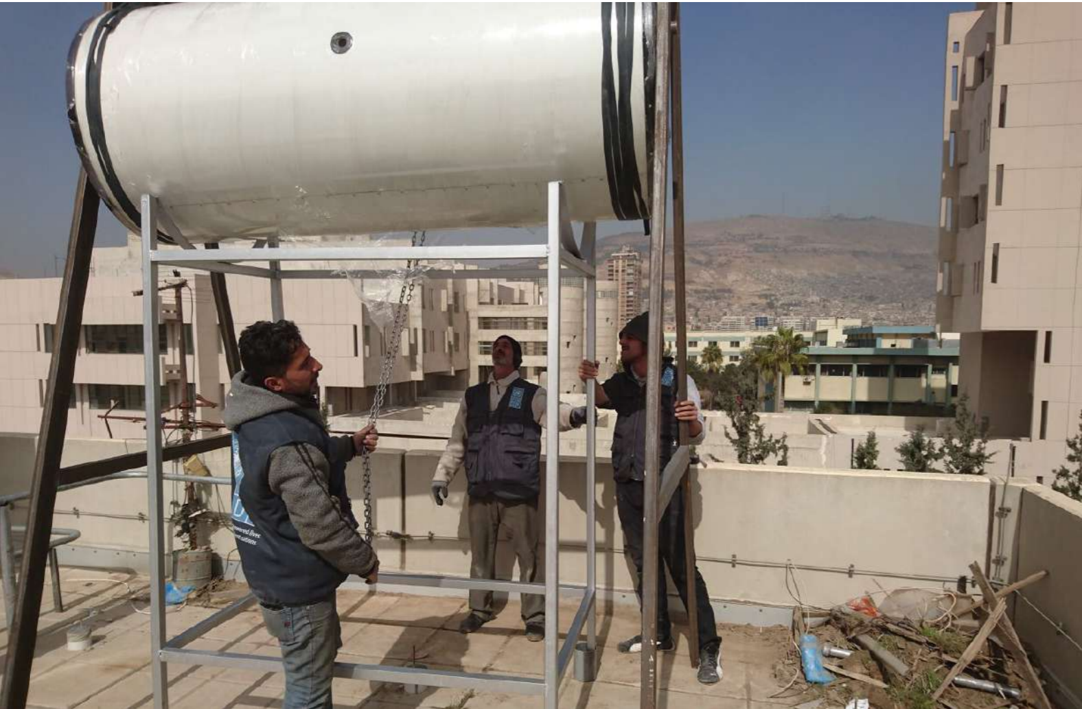
Installation works of solar heating units in the University Hospital in Damascus ©UNDP-Syria
